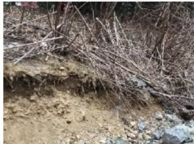
FIG 12: Erosion of Left Bank (Downstream Terminus of Existing Conveyance Channel, Upstream of Outfall)
