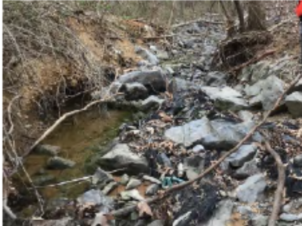
FIG 13: Observed Bank Erosion Upstream of Outfall (Facing Upstream)
