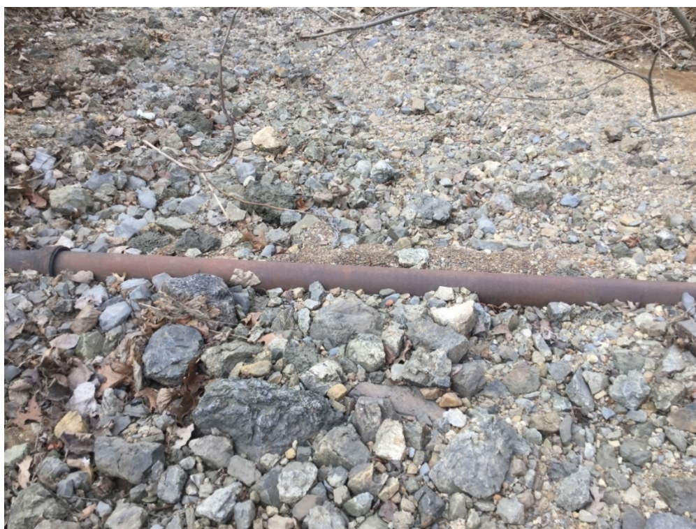
Figure 3-8 Exposed pipe in Reach 2 (6+75)
