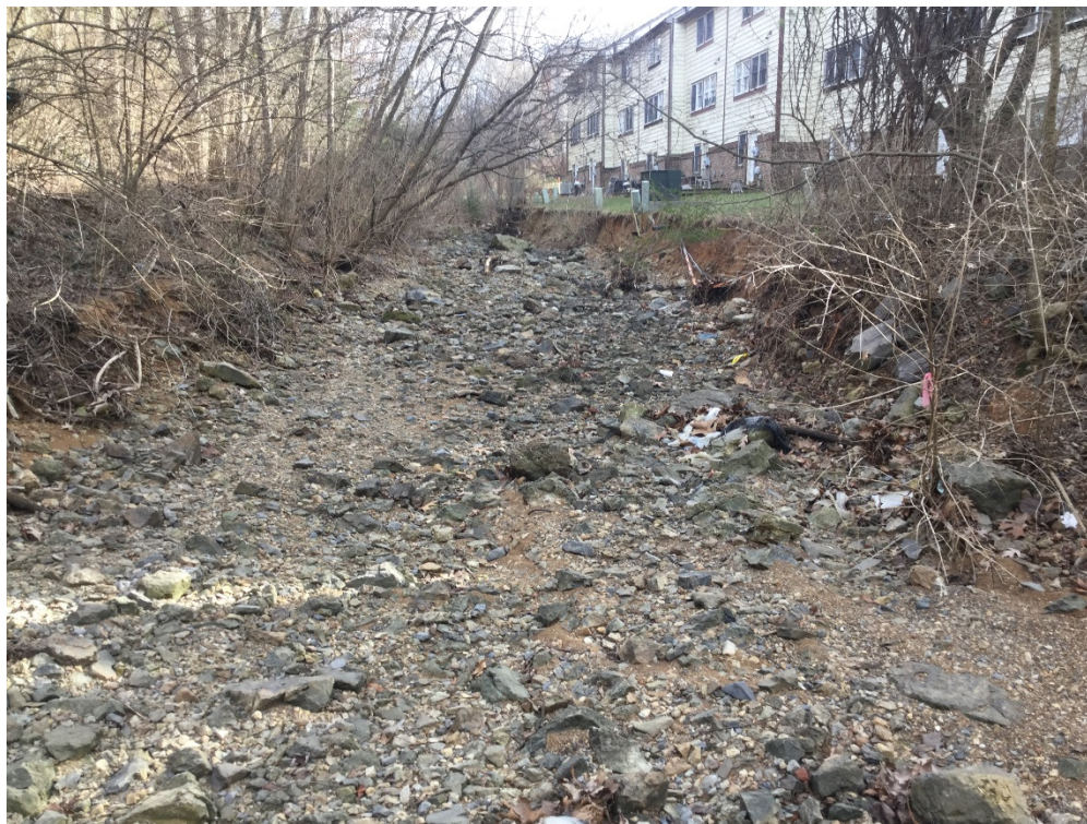
Figure 3-9 Looking up stream at eroding channel along Reach 2 (8+00)
