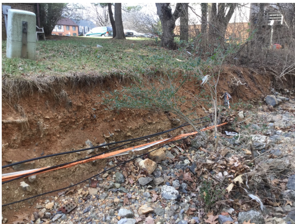
Figure 3-12 Exposed utilities along eroding bank (8+00)
