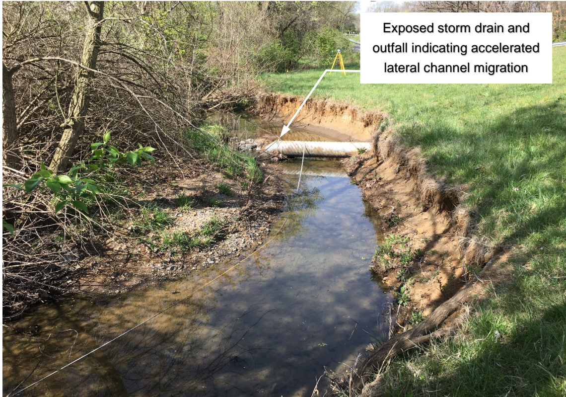
Figure 3-4 Eroded Streambank Meander Bend/exposed Pipe Along Reach 1
