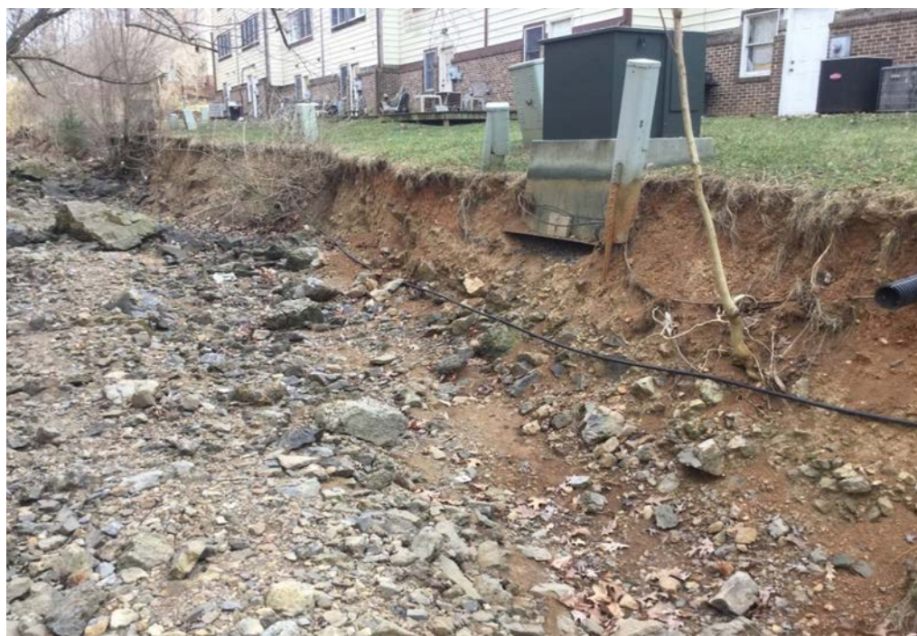
Figure 3-10 Looking upstream at eroding banks and exposed utilities along Reach 2 (7+50)
