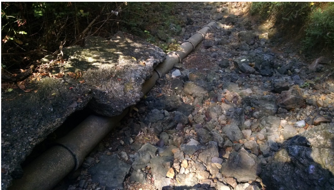
Figure 3-7 Exposed sewer line through stream section (6+00)
