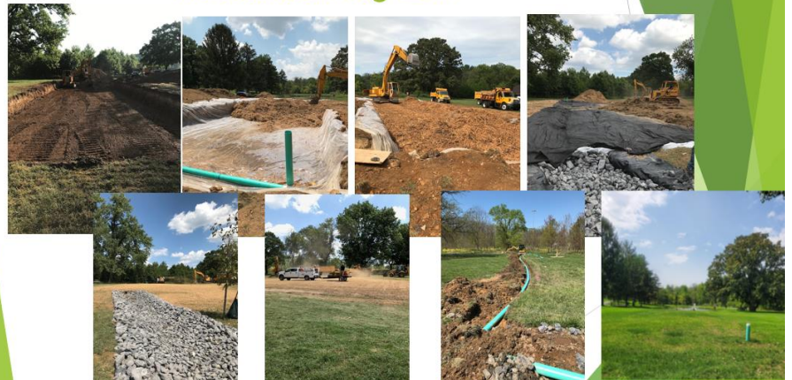
(Above) A collage of photos showing the installation of the Purcell Park Bioreactor Project.
