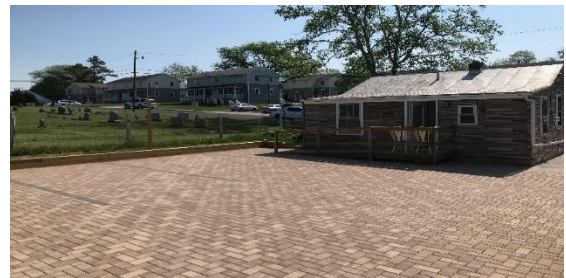
Permeable pavement allows stormwater runoff to filter through voids in the pavement surface into an underlying stone reservoir, where water is temporarily stored or infiltrated into the ground.
