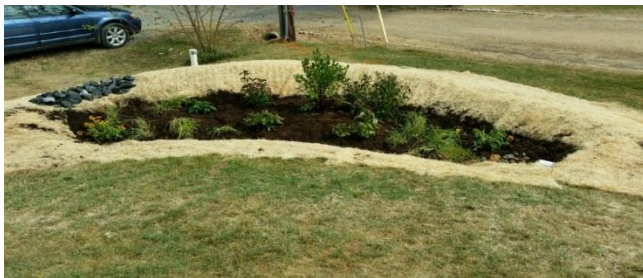
Rain gardens are shallow landscaped depressions that collect and remove pollution from stormwater runoff before it is infiltrated.
