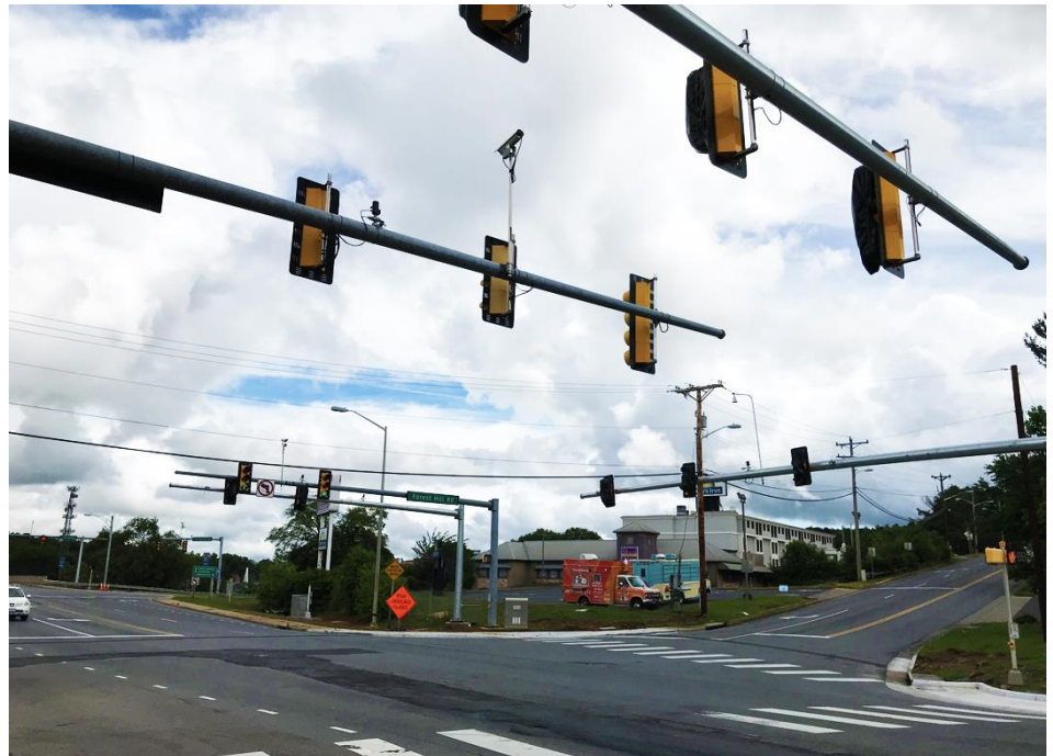
(Above) Signals at the intersection of Port Republic and Forest Hill roads will be changed over on Tuesday, June 23. Drivers will see lane closures during work.
