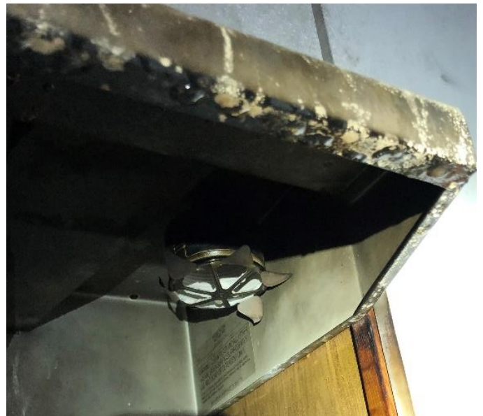
(Above) This Stovetop Firestop device helped stop a fire that recently occurred in Harrisonburg.
