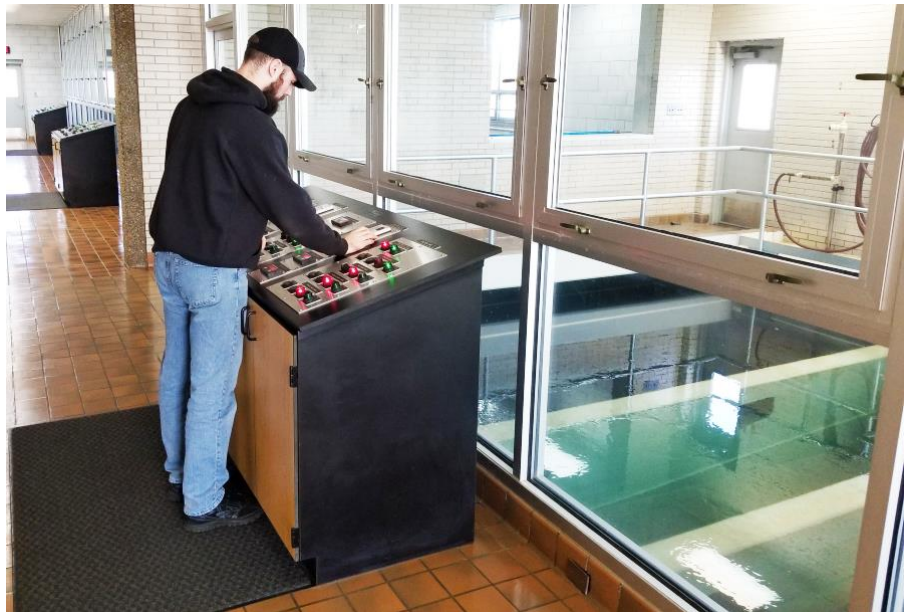
(Above) Operator Kyle VanOrden with the Harrisonburg Water Treatment Plant works at a filter system. The team recently received a Silver Award from the Virginia Department of Health's Office of Drinking Water for their work.
