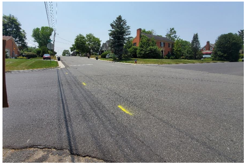
(Above) The first of two mini roundabouts will be installed at the intersection of Maryland Avenue and South Dogwood Drive starting Tuesday.
