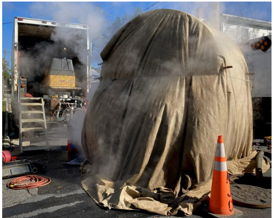
(Above) A thermally heated PVC pipe is inserted into the host pipe, and then pressurized so it expands tight against the existing pipe, eliminating the leaks while providing nearly the same capacity as the older pipe.
