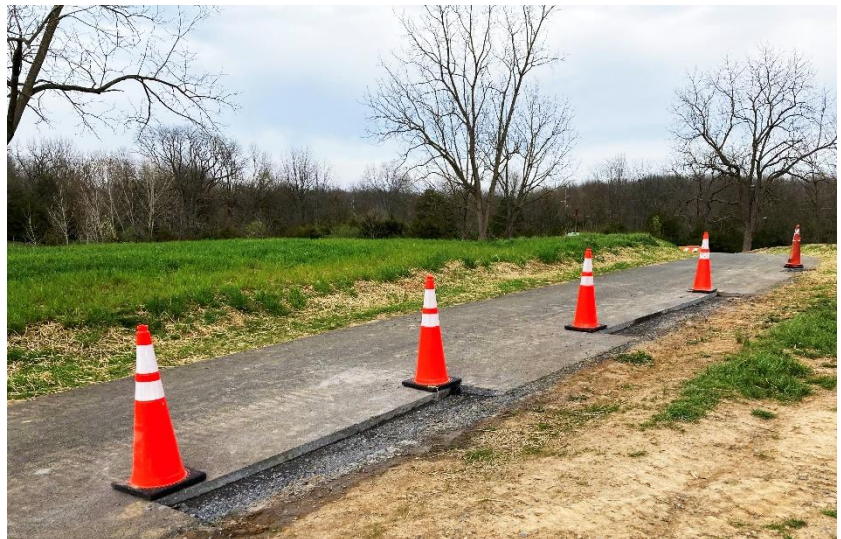
Patrons are asked to please avoid using the Friendly City Trail (above) starting Friday due to work scheduled to take place in the coming days.
