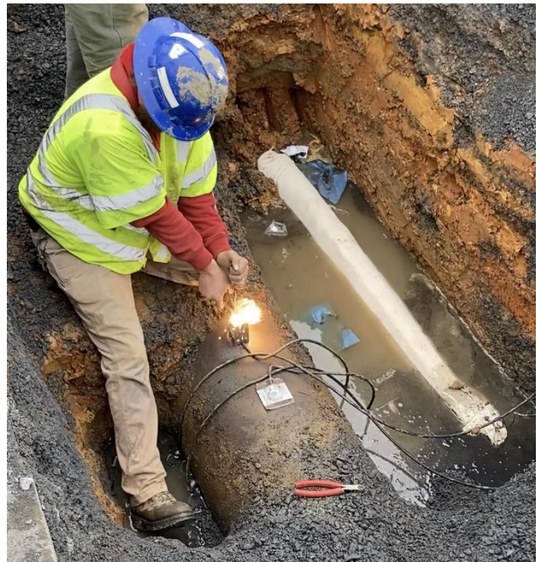
(Above) Harrisonburg Public Utilities Technician II Lincoln McQuillan welds a line connecting a water pipe to a magnesium anode.
