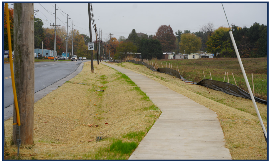
(Above) Sidewalk was constructed on the south side of Country Club Road between Linda Lane and Spotswood Homes mobile home park. A signalized crosswalk also was installed at Linda Lane to provide a safe route for walking from this neighborhood.
