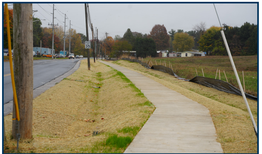
(Above) Sidewalk was constructed on the south side of Country Club Road between Linda Lane and Spotswood Homes mobile home park. A signalized crosswalk also was installed at Linda Lane to provide a safe route for walking from this neighborhood.
