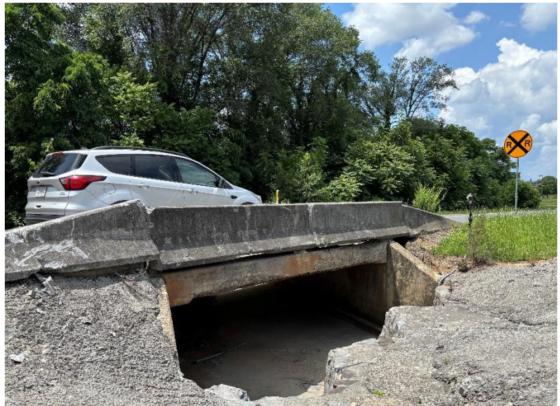
(Above) A culvert crossing on Country Club Road will be given a weight limit of 33 tons in the coming days.
