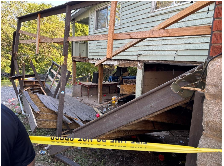
(Above)A deck connected to a Harrisonburg home collapsed on Monday afternoon, injuring several. Officials are urging community members to be mindful of safety when hosting events with large amounts of people attending.
